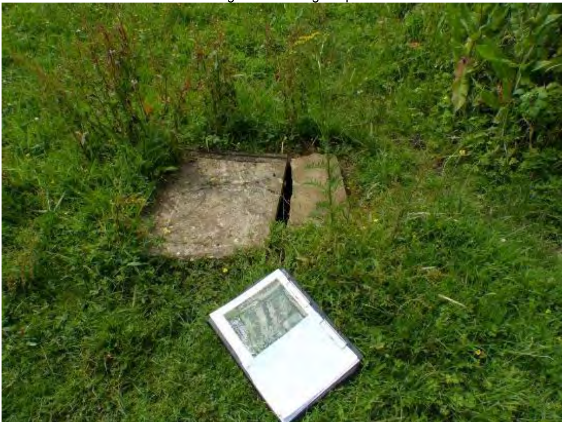
Photo A5.2: Broken cover over underground drainage in parcel 6.
